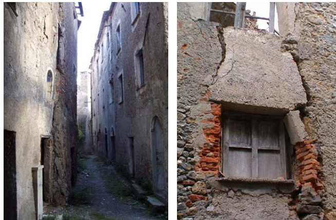
Figure 4: Inclination of the external walls (on the left); local buckling of the lintels (on the right).
