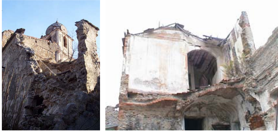
Figure 3: Masonry shattering (on the left) and internal collapses with vegetation growth (on the right).
